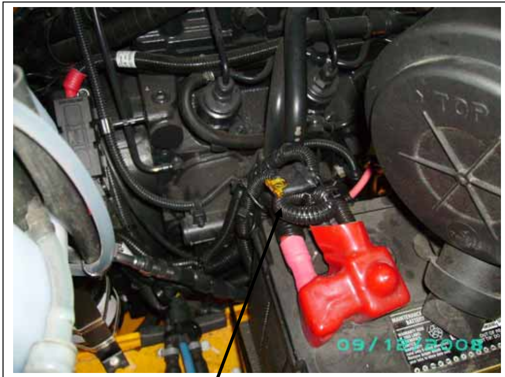
Power from battery through ATO fuse to relay.
