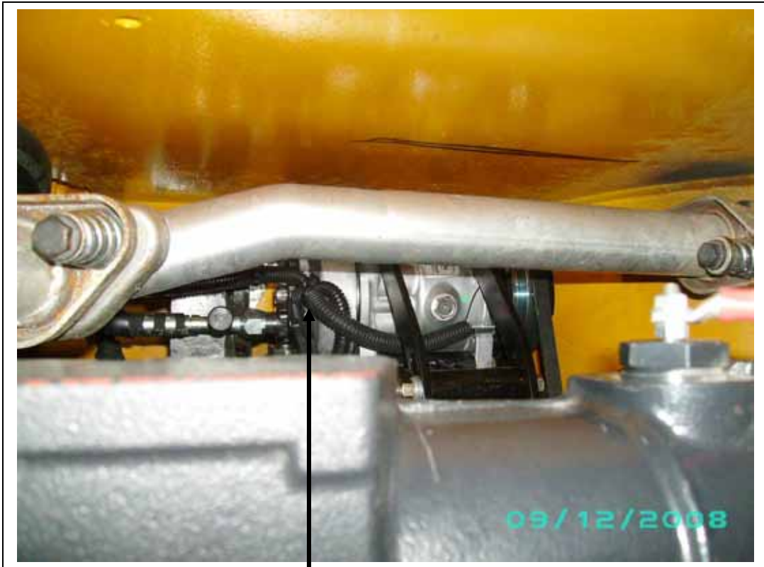
Electrical connections at compressor. Wire in to binary then out to the compressor clutch.
